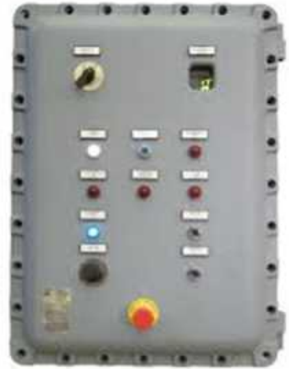
ATEX Electrical Control Panel
